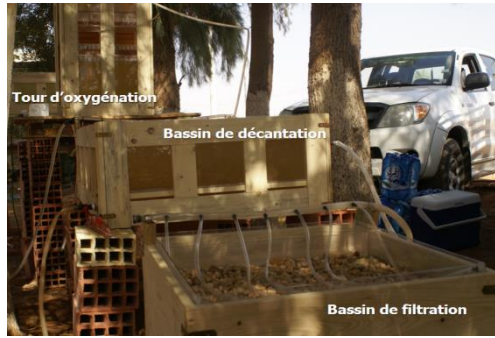
Fig 5: iron removal station by natural oxygenation (TDF)
