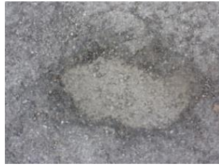
Fig.13. Left image of Pothole
