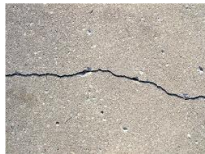
Fig. 2. An RGB image of a crack
