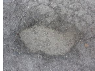
Fig.14. Right image of Pothole
